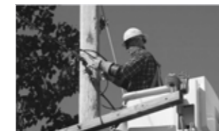
LV overhead networks
