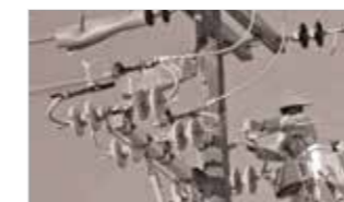
MV overhead networks
