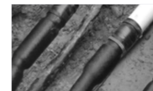
MV underground networks
