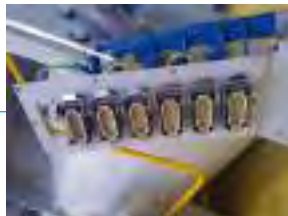
■ High-tension switch cabinet
