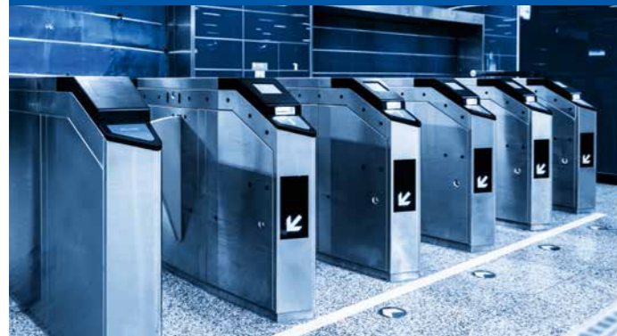
Ticketsysteme / Ticket systems
