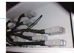
In control system
